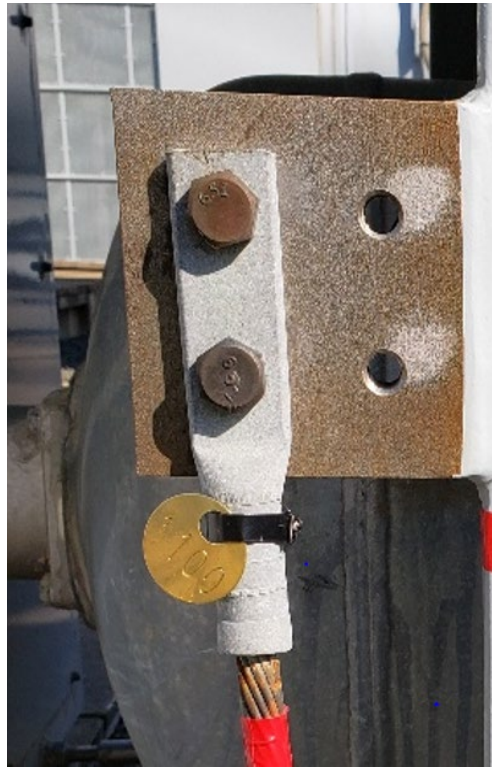
FIG. 5 – Example of Labeling Ground Risers from Client Site
