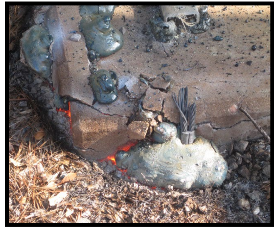
FIG. 4- Copper Theft (Cut Ground on Regulator Neutral)
