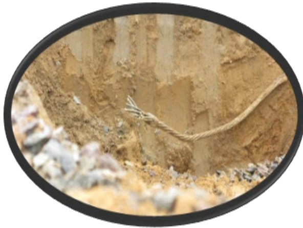
FIG. 3 – Broken 4/0 Copper Conductor at Client Site
