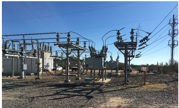
Lakeshore Substation pre-modernization
